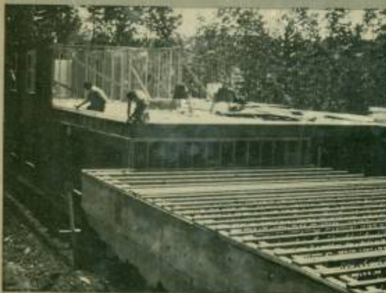
The Lambda Chi house continues to rise as Alfred brothers Jim Rausch and Greg Young work on the second floor.
